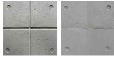
10 mm Grouting No Grouting
